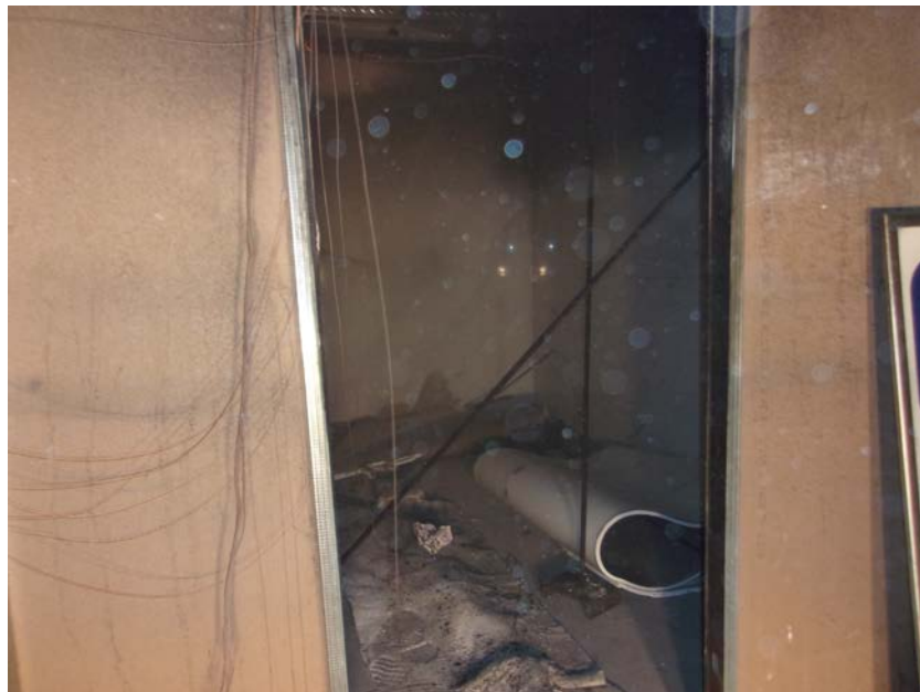
Middle ceiling panel falls
