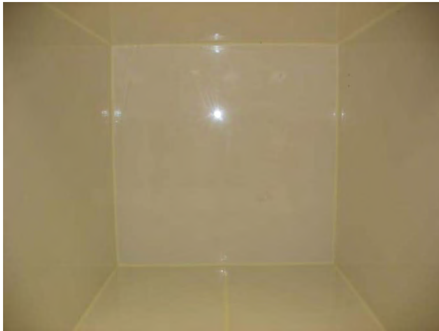
Photo No. 3 Interior View of Chamber Showing Corner and Butt Joint Seams
