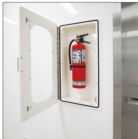
Fire extinguisher cabinets
